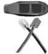
Wrong Wiring but Functional
